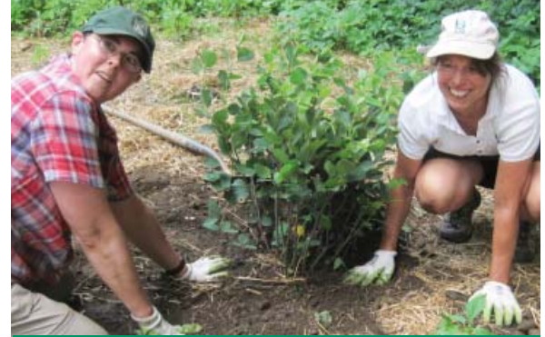
Volunteer Sharon Siter (left) and HVA Berkshire Outreach Program Manager Alison Dixon plant a rain garden next to the new culvert on Churchill Brook.
