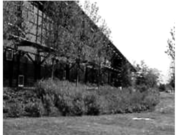
Rooftop without gutters!
